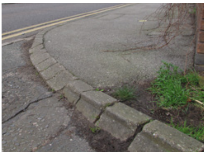
Inappropriate dropped kerbs
