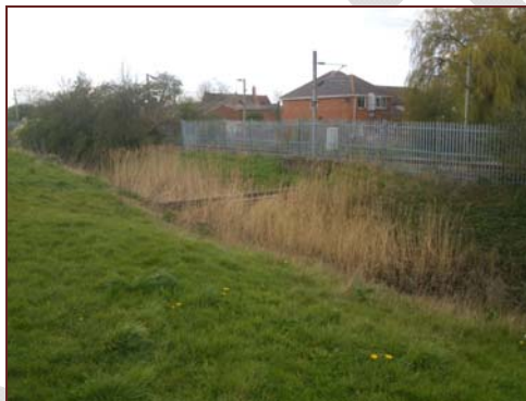
FIGURE 3: EAST DOCK SEWER, OVERGROWN VEGETATION
