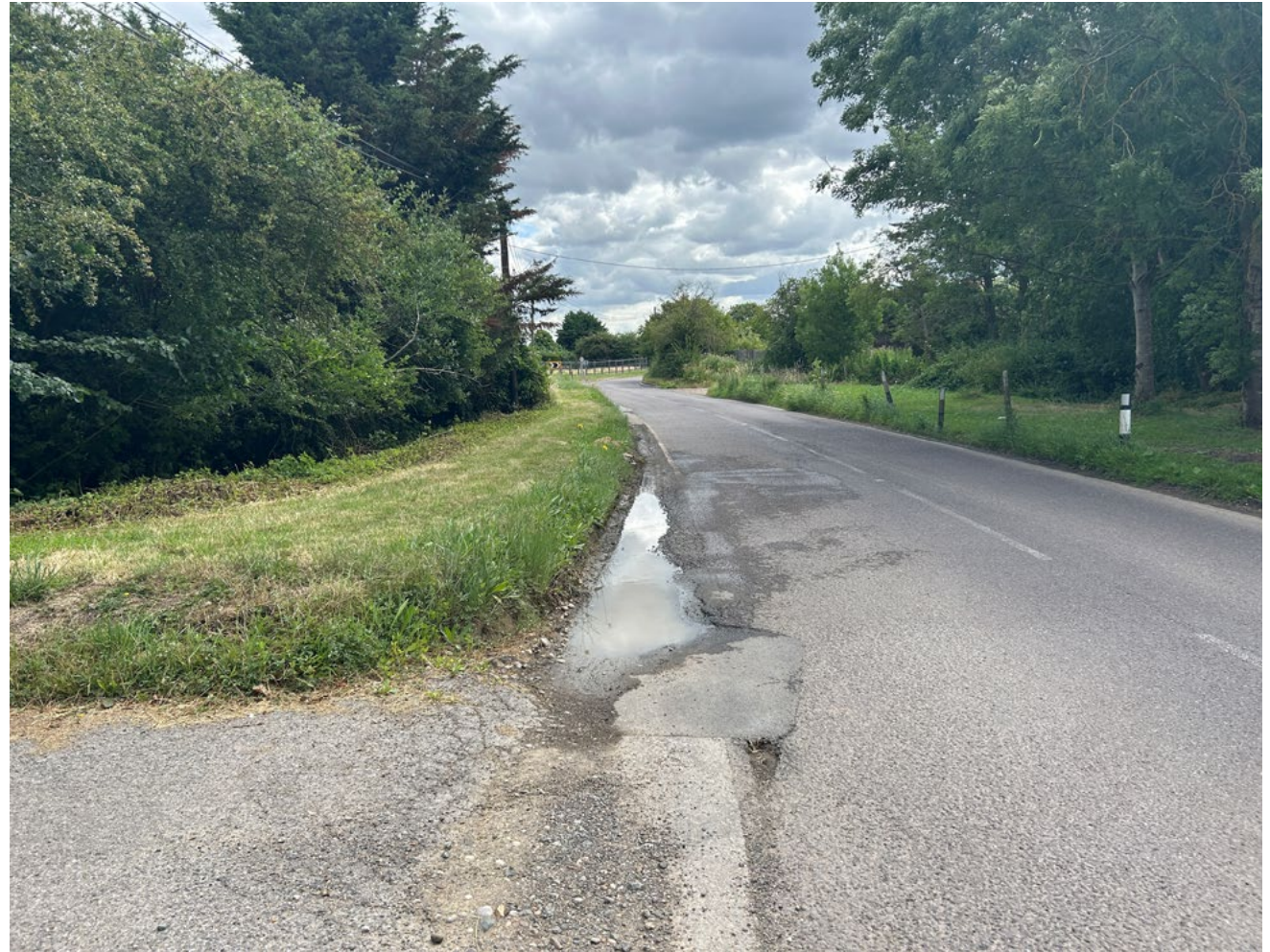
Fig 79. Surface water flooding in July on Fen Lane
